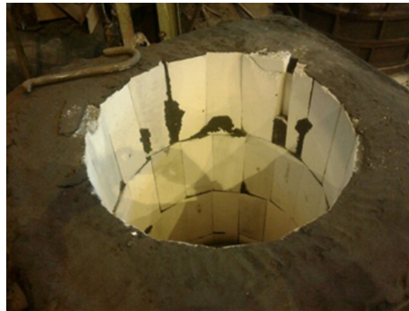
Figure 1. Layer of ceramic bricks built as isothermal cleading of a riser head
